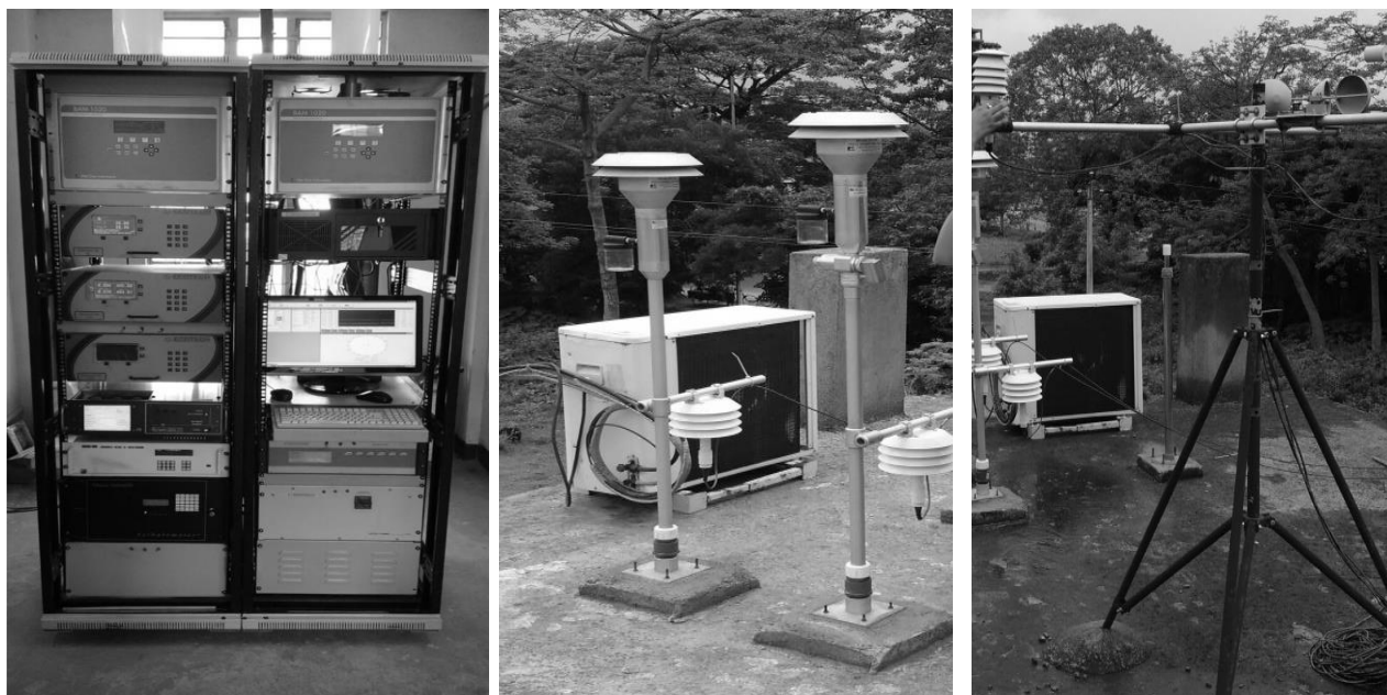
Fig: 1 Echo Tech Serinus 30 Carbon Monoxide Analyzer (Pollutants detector, pm 2.5 & pm 10, wind direction & wind speed sensor)
